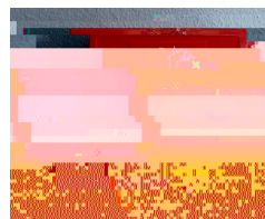
Fire alarm call point
